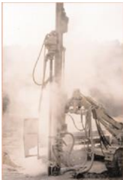
(Source: HSE Dust and silica – reproduced under the terms of the Click-Use licence) Figure 10.6 – Crawler mounted drill with no dust control
